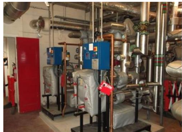
One of the new units
