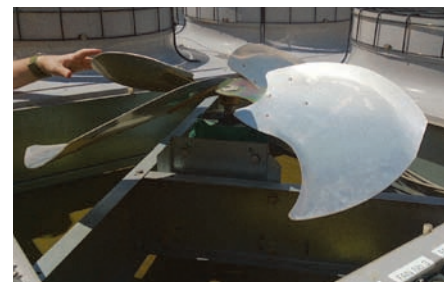
Figure 2: The datacentre’s existing AC fans were nearing the end of their useful life
